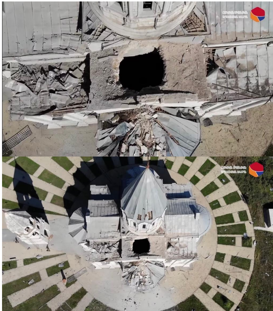
Figure 21: The damaged roof of the St. Holy Savior Ghazanchetsots Cathedral from outside after the second strike
