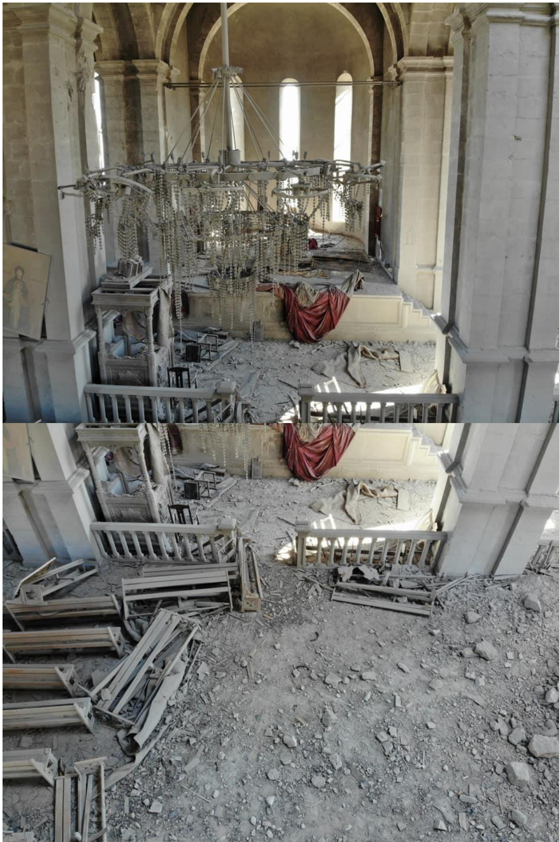
Figure 22: The damaged roof of the St. Holy Savior Ghazanchetsots Cathedral from inside after the second strike
